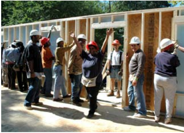
Volunteers raise the walls of the Habitat for Humanity house in Atlanta near the beginning of the project.
